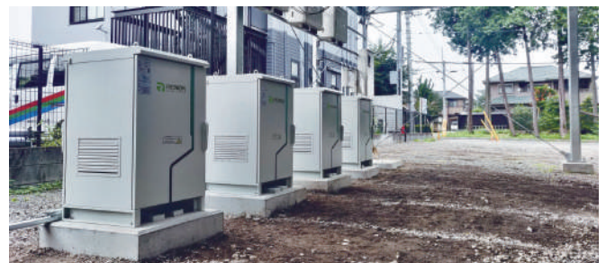
Renon DC ECube 15kWh
