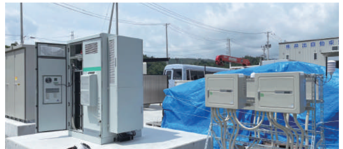
Renon DC ECube 157kWh
