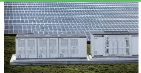
Industrial Electricity Generating Station
