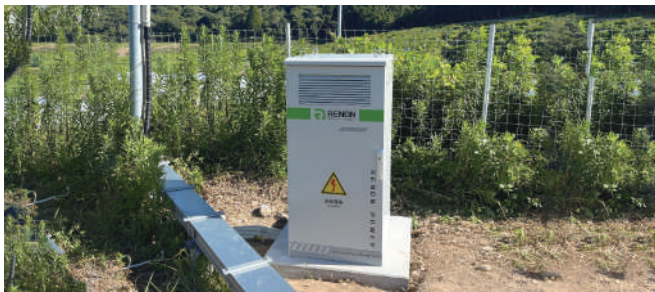
Renon DC ECube 38kWh
