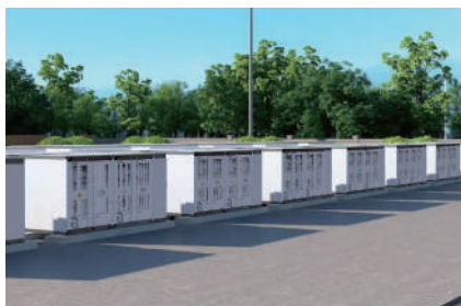
ELECTRICITY GENERATING STATION
