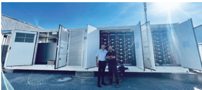
Renon Estation 744kWh
