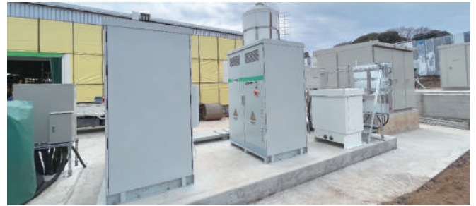
Renon DC ECube 157kWh
