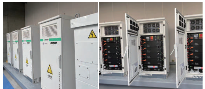
Renon DC ECube 38kWh
