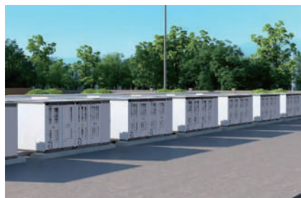
ELECTRICITY GENERATING STATION
