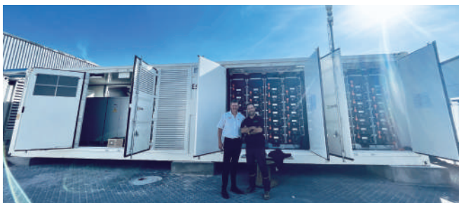
Renon Estation 744 kWh
